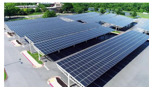
■ 澳门光储充一体化车棚 Macao PV-ESS-EV Charging Carport
