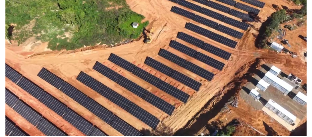
■ 斐济海岛, 光储柴系统, 纯离网系统, 1.7MW光伏配1.5MW/2.98MWh储能 Fiji Island, light fuel storage system, pure off-grid system, 1.7MW PV with 1.5mw/2.98MWh energy storage
