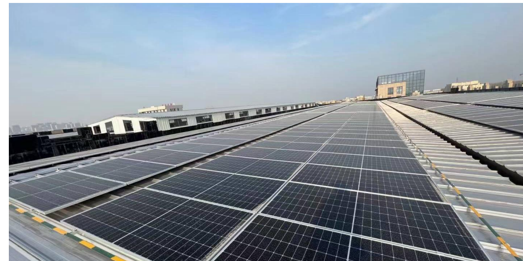
■ 越南同奈省纺织工厂4.7MWp屋顶 4.7 MWp Rooftop Solar Project at a Textile Factory in Dong Nai Province, Vietnam
