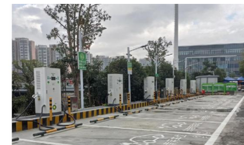
■ 宁波-清水桥菜市场光储充一体化充电站 Ningbo Qingshuiqiao Vegetable Market PV-ESS-EV Charging Station
