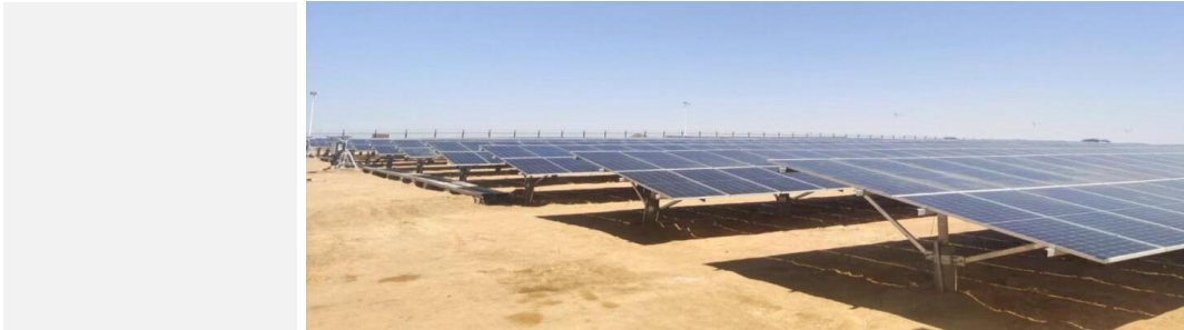
■ 乍得光储项目, 3.6MW光伏配2.5MW/7.776MWh储能 Chad PV plus energy storage project, 3.6MW PV with 2.5MW/7.776MWh energy storage
