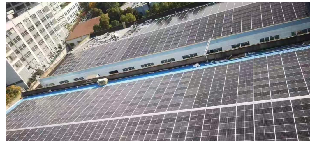
■ 越南头顿鞋厂3.6MWp屋顶 3.6 MWp Rooftop Solar Project at the Vung Tau Shoe Factory in Vietnam
