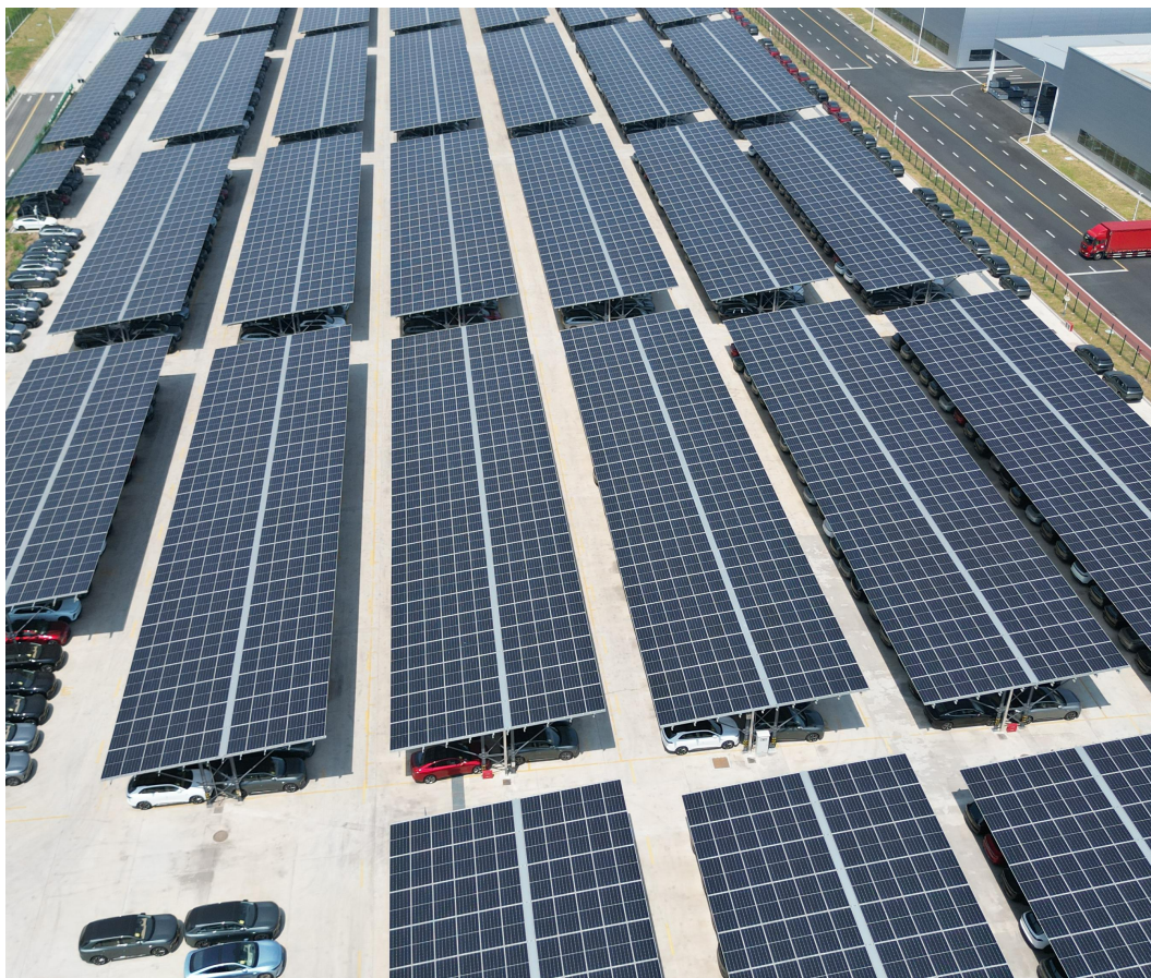
■ 芜湖奇瑞物流园4.2MWp光伏车棚项目 Wuhu Chery Logistics Park 4.2MWp PV project
