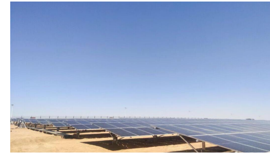
■ 乍得伊里巴光伏2.5MW+储能7.776MWh项目 Chad Iriba 2.5 MW Solar Power + 7.776 MWh Energy Storage Project
