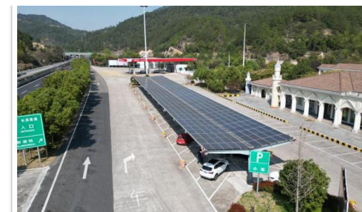
■ 长深高速服务区光储充一体化车棚 Changshen Expressway Service Area PV-ESS-EV Charging Carport
